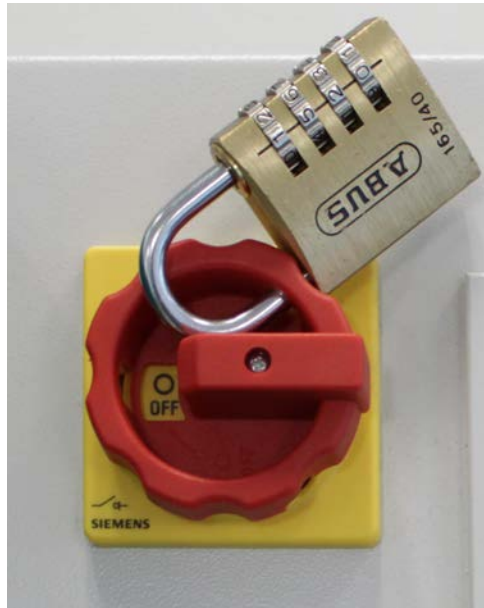
Fig. 2: Electrical main switch protected with a padlock
