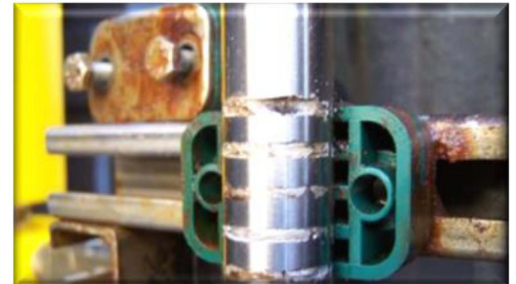
Fig 1 – Tube showing signs of crevice corrosion
